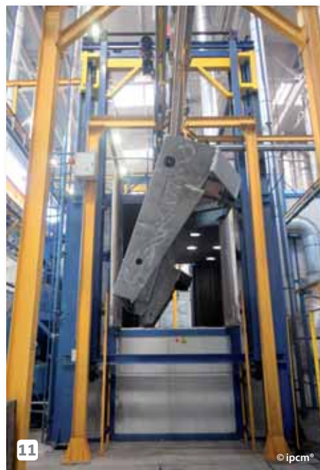
11 The shot blasting system. La granigliatrice.
