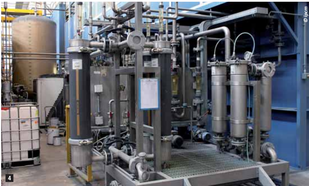
4 The ultrafiltration module installed by Verind with 8 inches spiral membranes.
